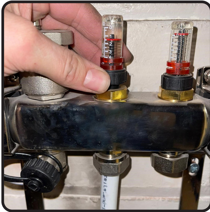
Flow meter open (collar removed)
